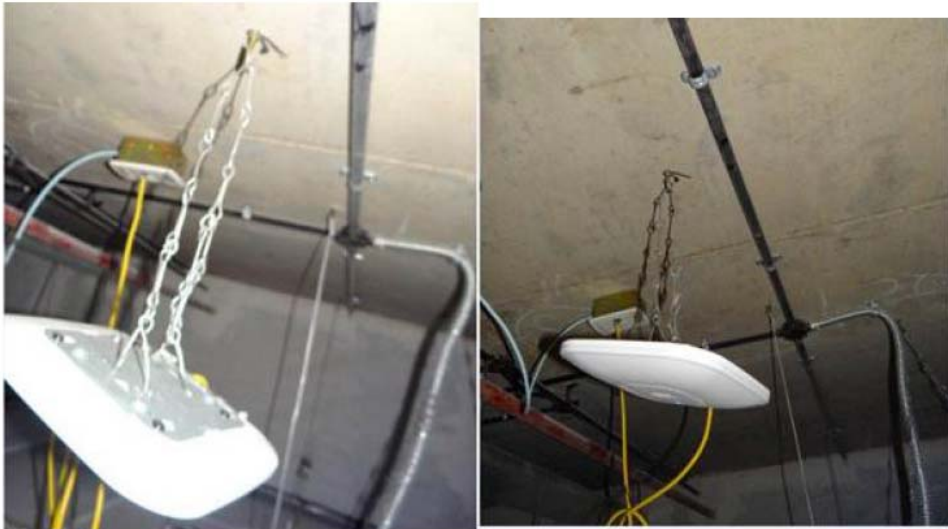
Figure 91 Example of a Poor Installation - Access Point Needs to be Level and Not Swing or Move About
