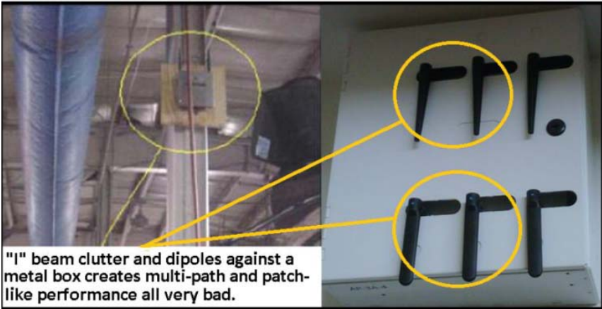
Figure 90 Example of an AP Installation Near Metal and Clutter (Again, Try to Avoid Metal and Clutter)
