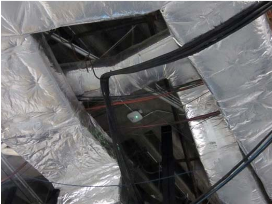
Figure 92 Example of a Poor Installation – Access Point is too High and Buried in Conductive Foil
