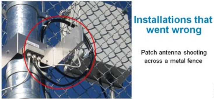
Figure 89 Patch Antenna Against a Metal Fence
