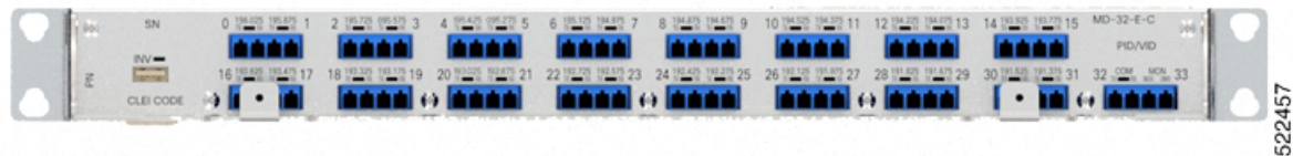
Figure 11: N1K-MD-32E-C Patch Panel Front View
