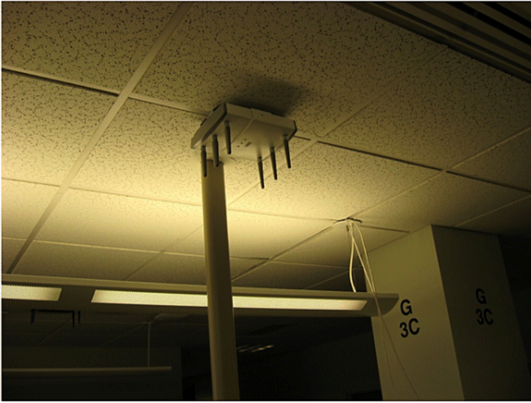
Figure 12: Poor AP Placement - AP Placed Near Physical Obstruction
