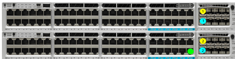
Dual 10/25GE ToR Switches (standalone or stacked)
