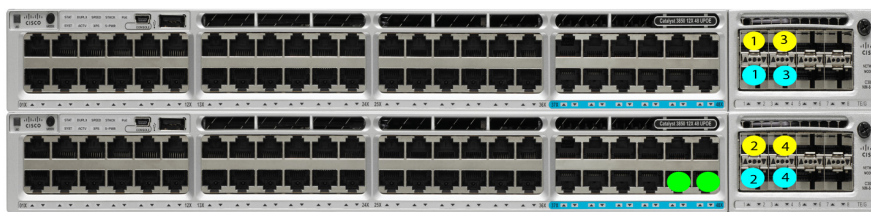
Dual 10/25GE ToR Switches (standalone or stacked)
